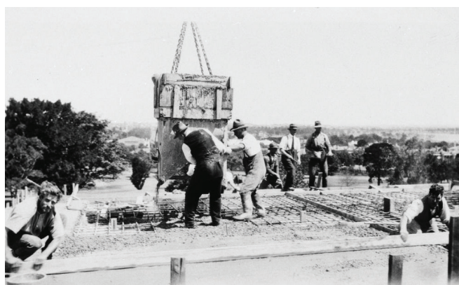
Workers pour and screen concrete on the south terrace c 1928–34 Shrine Collection
