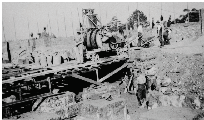
Concrete team spading the foundation trenches down to the bedrock c 1928 Shrine Collection
