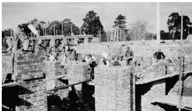
Bricklayers forming piers for the foundation of the main structure c 1928–34 Shrine Collection
